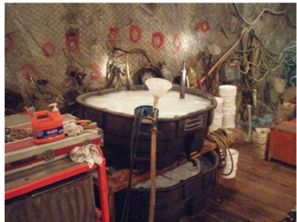
Figure 15. Dry Synthetic Mud Mixing System
