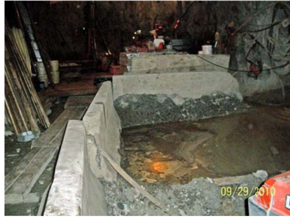
Figure 13. Mud Sump Showing Precipitated Mud
